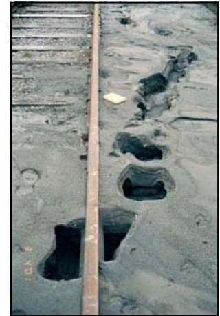
Liquefaction in action; this photo shows sand being ejected through a crack subsequently forming a chain of sand boils in Olympia Washington (Source: U.S. Department of the Interior, U.S. Geological Survey)
