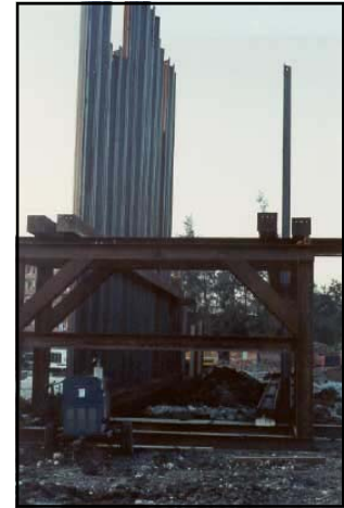
Sheet pile template; these horizontal beams provides inside and outside support near ground level (Source: Pile Branch® Inc.)
